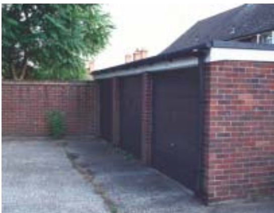
Rear parking – Poor surveillance, poor quality
